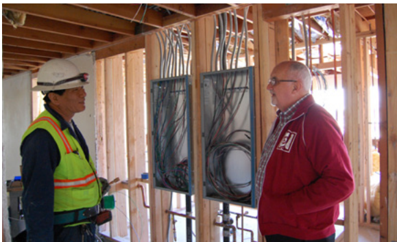
Jong the electrician speaks to Fr. Tim Ploch about the electrical panels
