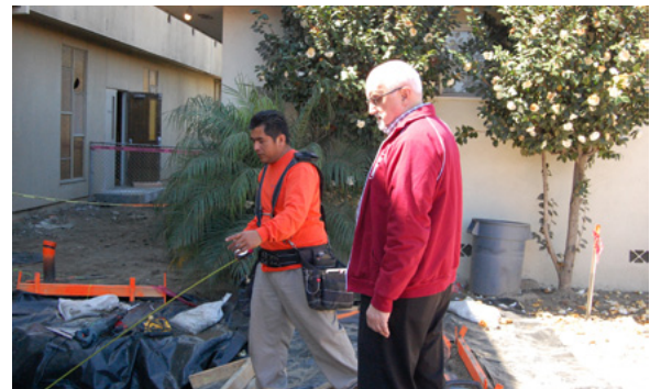
Alfredo Urbina explains the forming of the elevator walls to Fr. Tim Ploch
